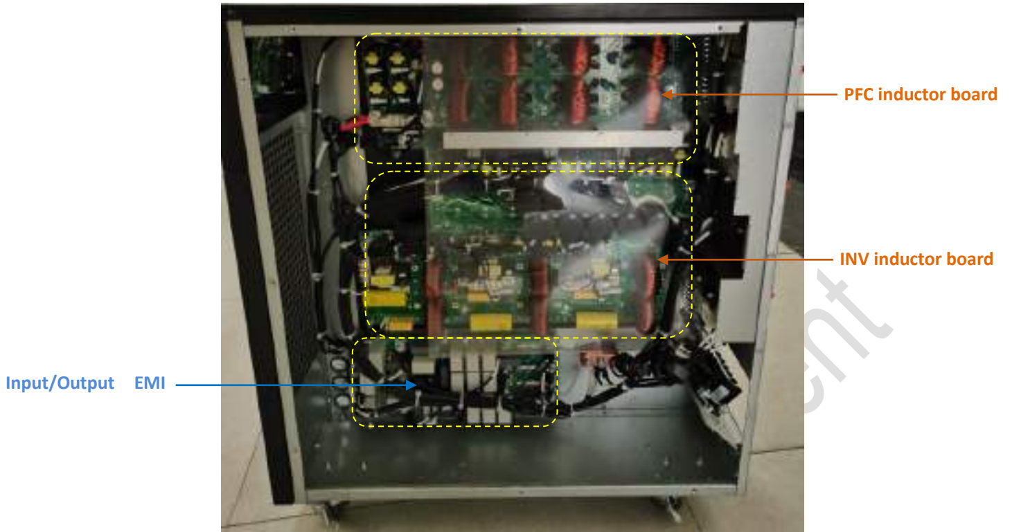
Figure 13. UPS right view (10K)
